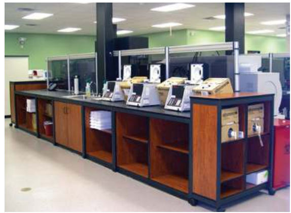
LAB ISLAND WITH INTEGRATED UTILITIES AT CELL WASHERS
